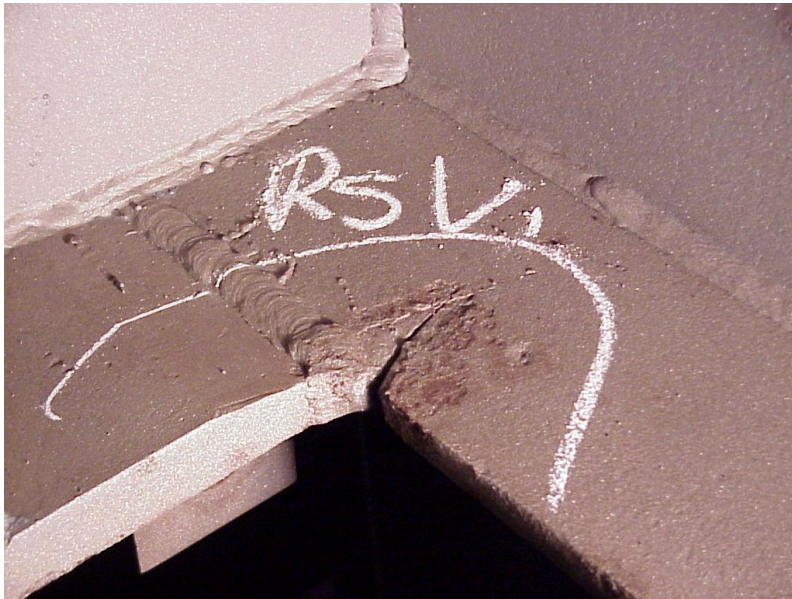
Cracks in Old Gates
