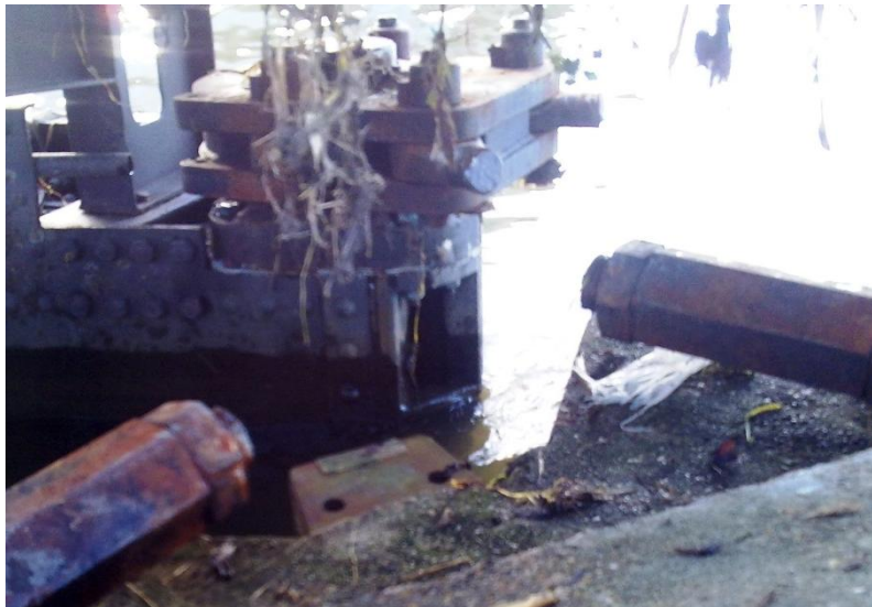
Anchorage failure due to low ductility of Steel ( Y_S < 1000 MPa is recommended)
